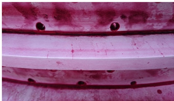
Figure 2: Indication shown on the hoop by Penetrant Testing
