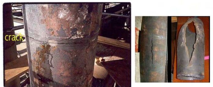
High temperature creep crack at weld (Brittle)
